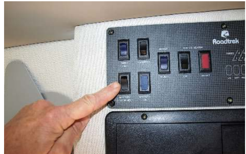
Battery disconnect switch
