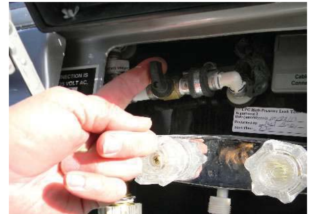
City water valve in shut position
