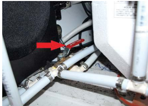
Tank selection valve in exterior tank position
