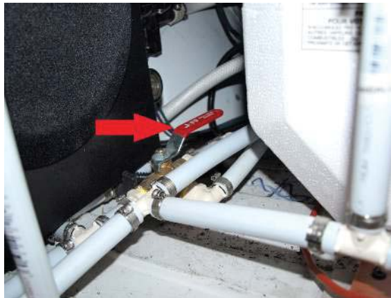
Tank selection valve in exterior tank position
