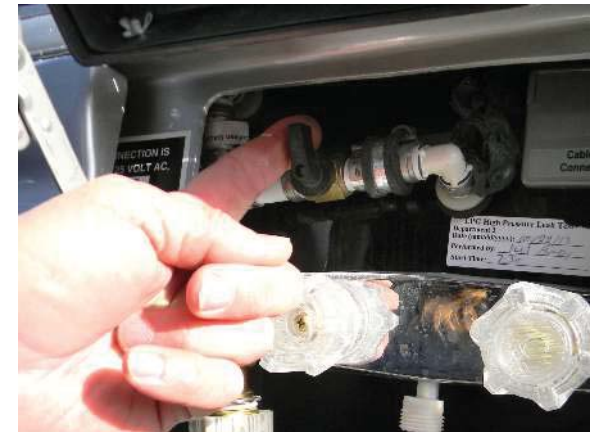
City water valve in shut position
