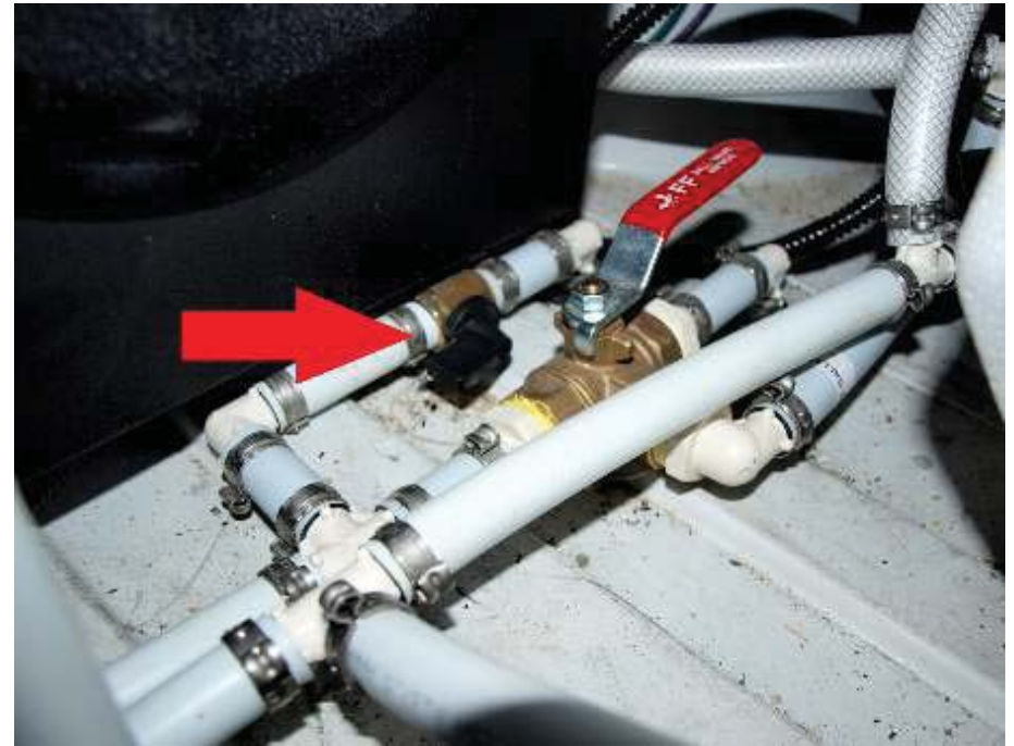
Tank isolator valve in open position
