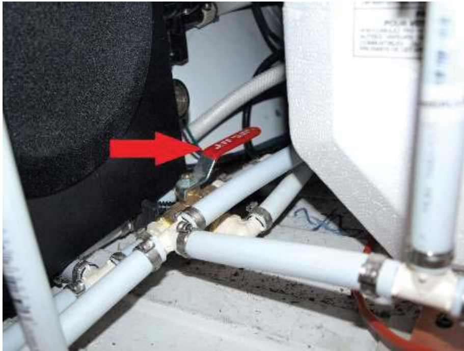
Tank selector valve in exterior tank position
