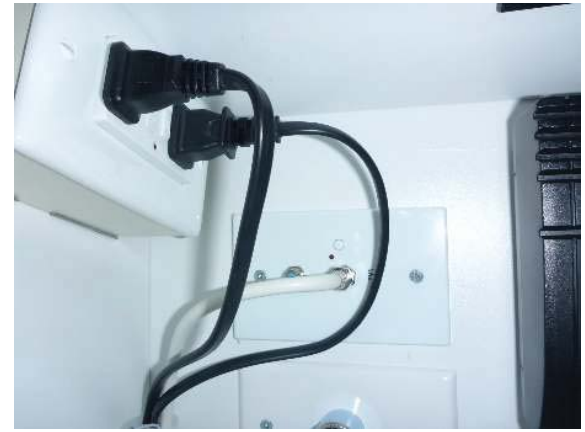
TV antenna switch
