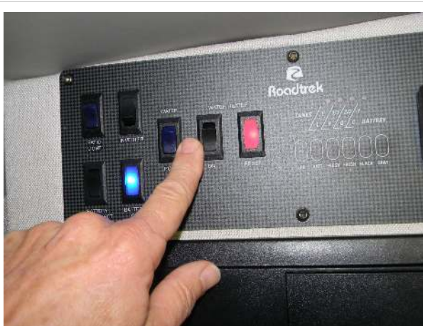
Water heater switch and red indicator light
