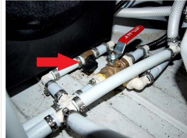
Tank isolator valve in open position
