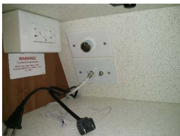
TV antenna and cable connections
