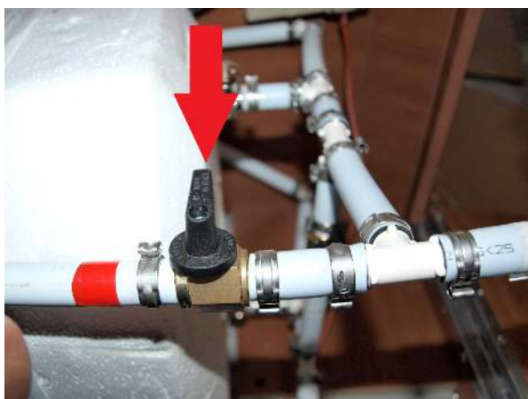
Hot water shutoff valve, shown closed
