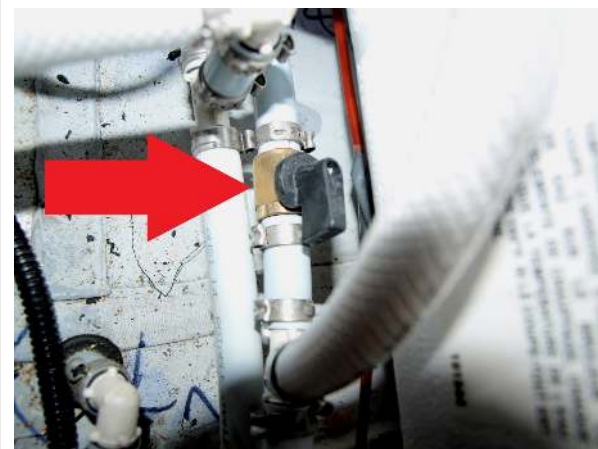
Cold water shutoff valve, shown open
