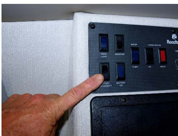
Battery disconnect switch
