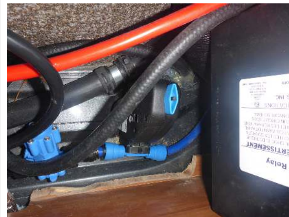
Resetting the tripped valve
