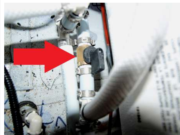
Cold water shutoff valve, shown open
