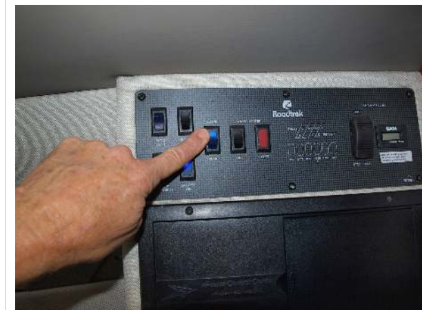
Water pump switch
