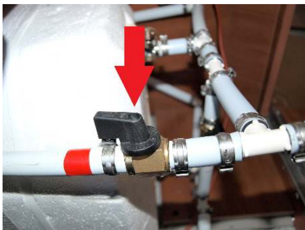
Hot water shutoff valve, shown open
