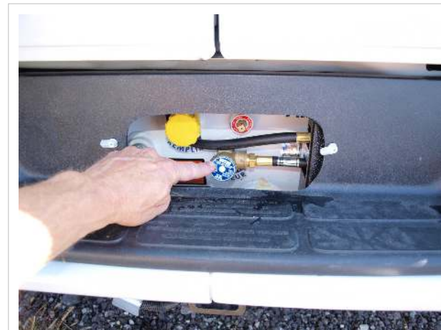
Propane tank main shutoff valve
