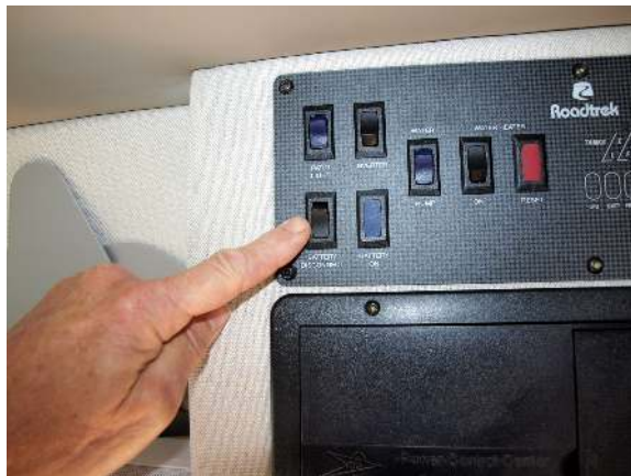
Battery disconnect switch
