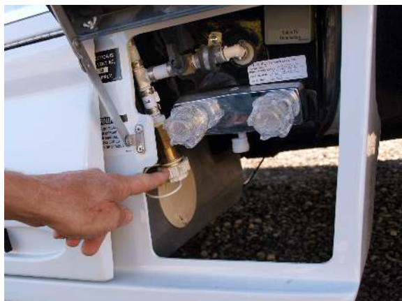
City water fill location
