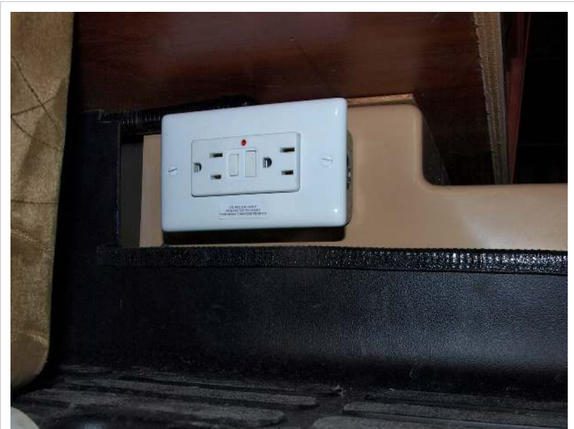
GFCI outlet under rear passenger side seat
