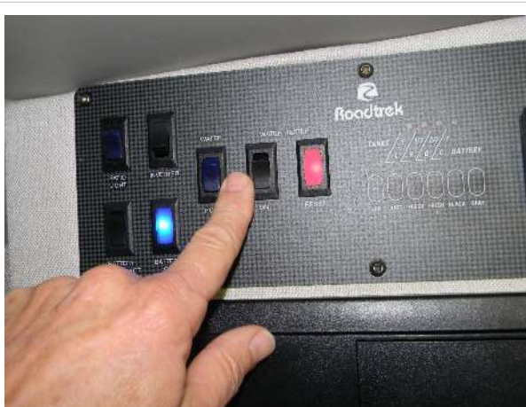
Water heater switch and red indicator light
