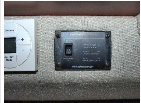
Inverter switch for big inverter
