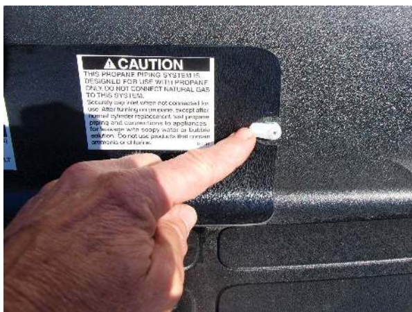
Propane tank cover
