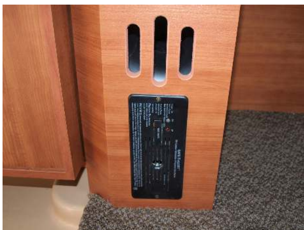
Propane and CO alarm
