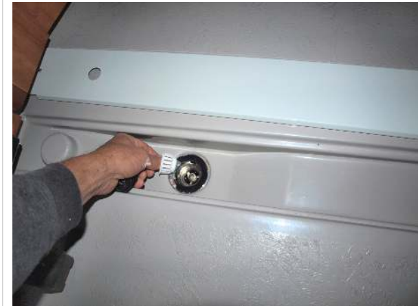
Aisle shower drain
