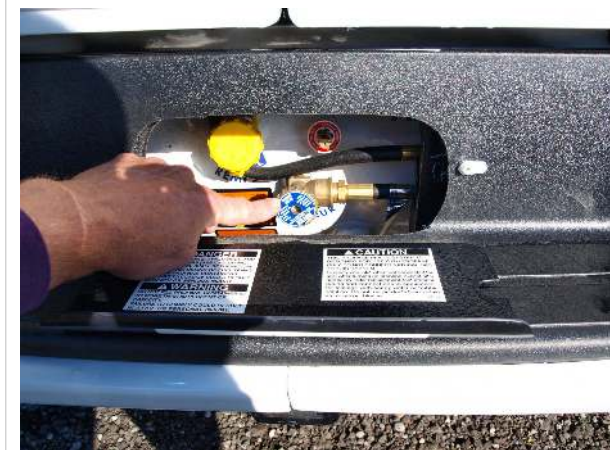
Propane tank main shutoff
