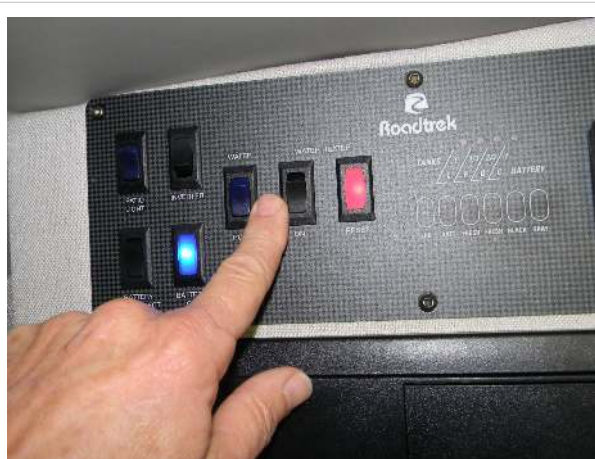
Water heater switch and red indicator light
