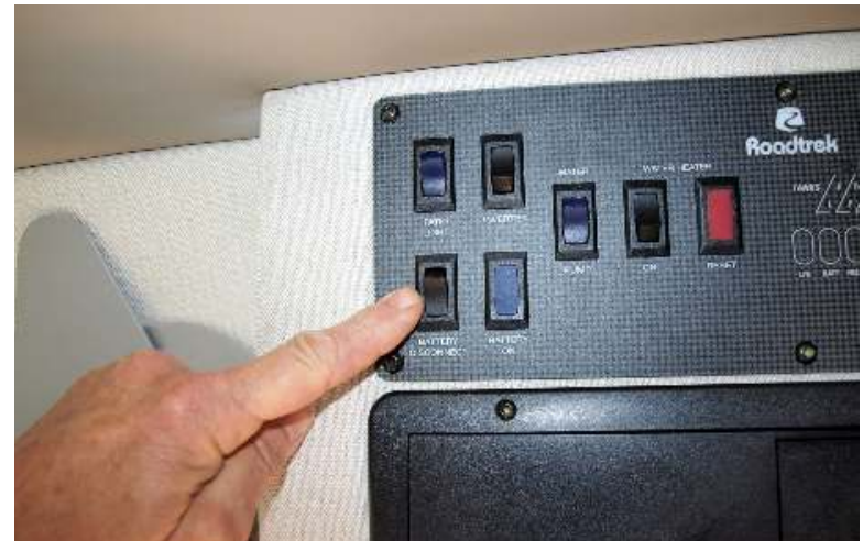
Battery disconnect switch
