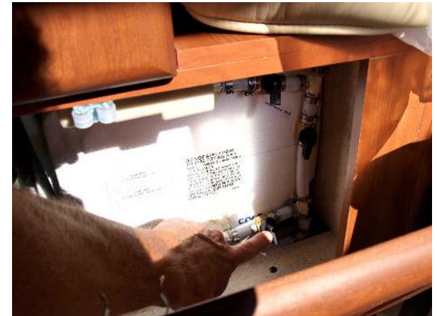
Water heater enclosure
