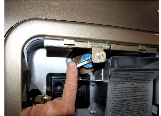
Water heater pressure relief valve
