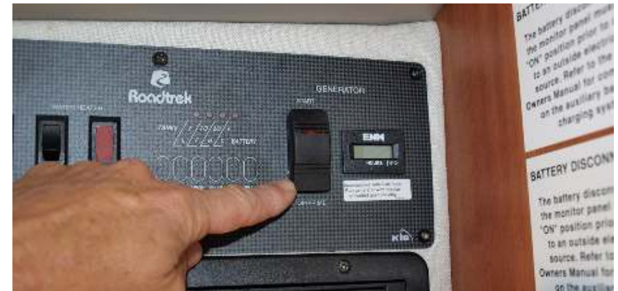
Generator switch, prime/off position
