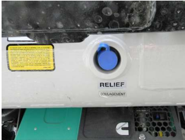
Propane relief valve
