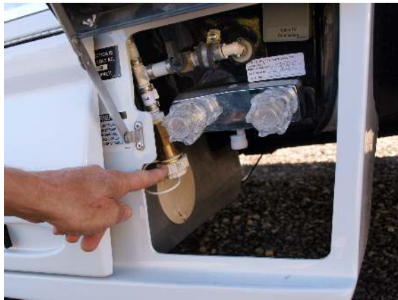
City water fill location
