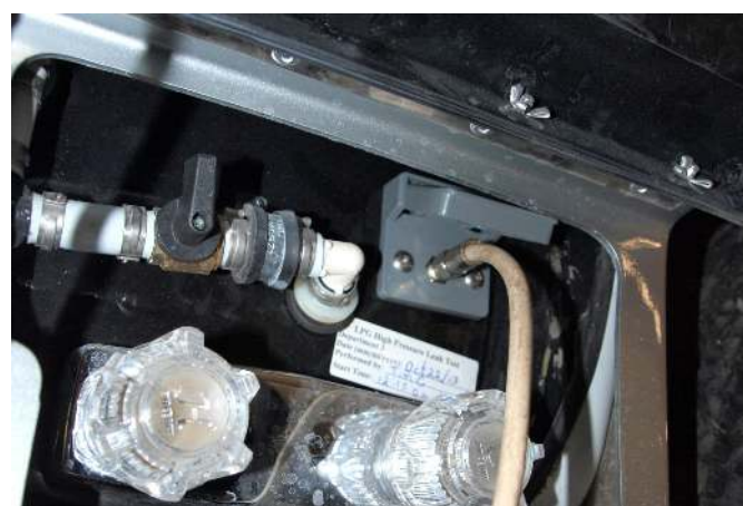
TV cable connected
