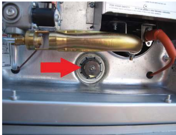
Water Heater Anode
