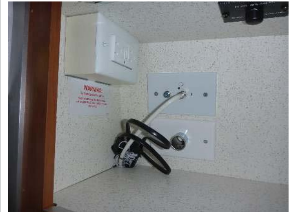
TV antenna switch (the small white button near the antenna connectors)
