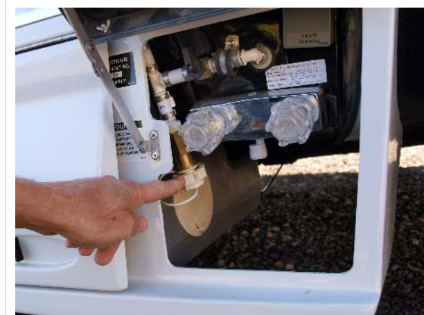
City water connection
