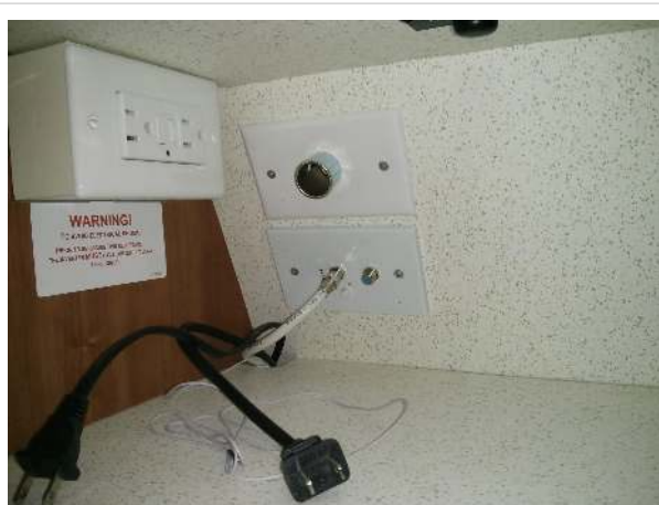
TV antenna and cable connections
