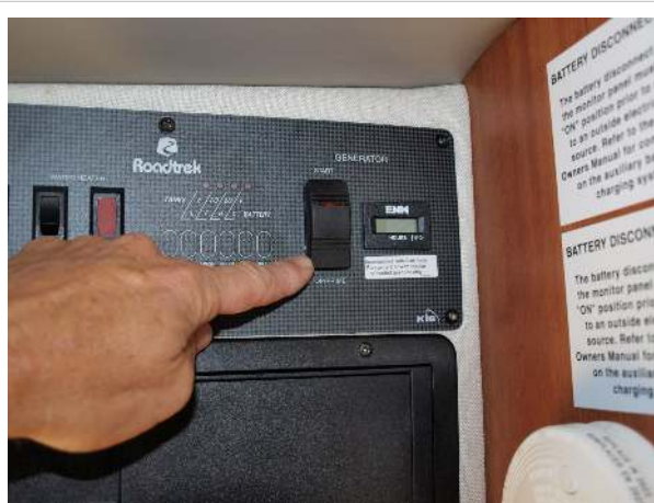
Generator switch, prime/off position
