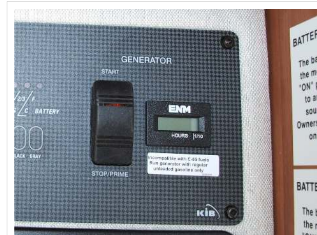
Generator switch and hour meter
