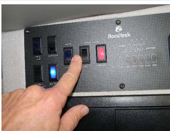
Water heater switch and red indicator light
