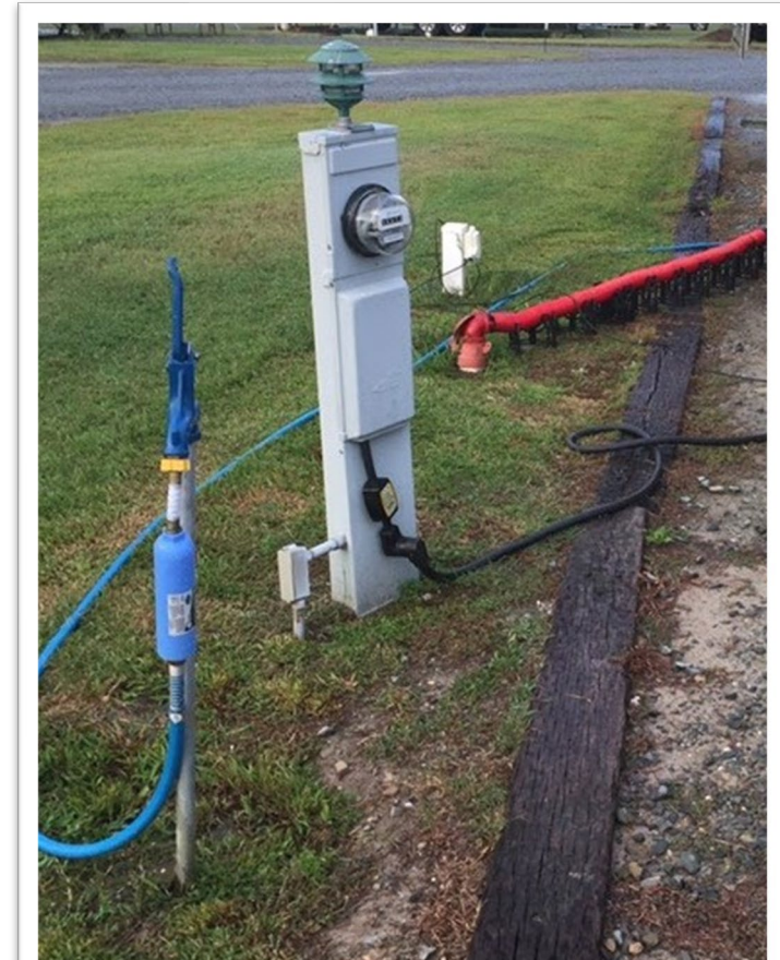
Full hookups - electric, water, and sewer
