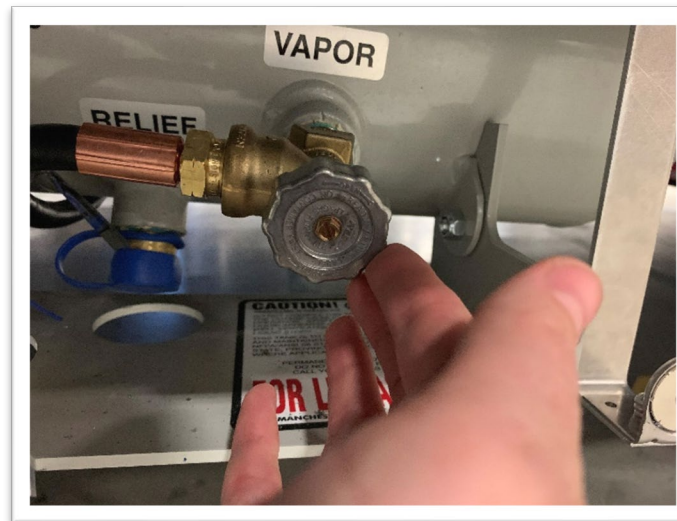
Propane tank main shutoff valve
