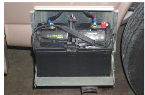
Picture B-P39: Auxiliary battery hex nut posts on top of battery
