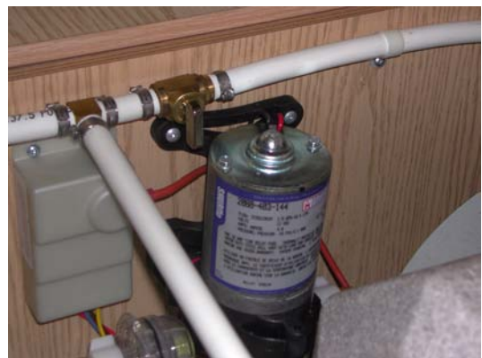
Picture G-P19: Hot water cutoff valve in closed position.
