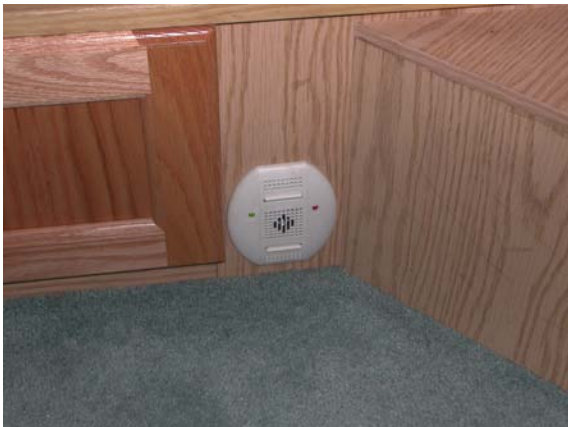
Picture F-P1: L.P.G. leak detector.
