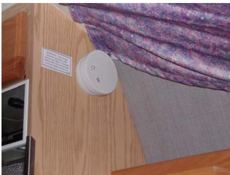
Picture F-P3: Smoke detector.
