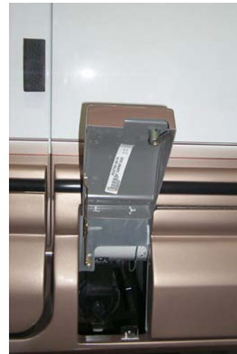
Picture G-P7: Access to sewer discharge assembly, black and grey gate valve handles
