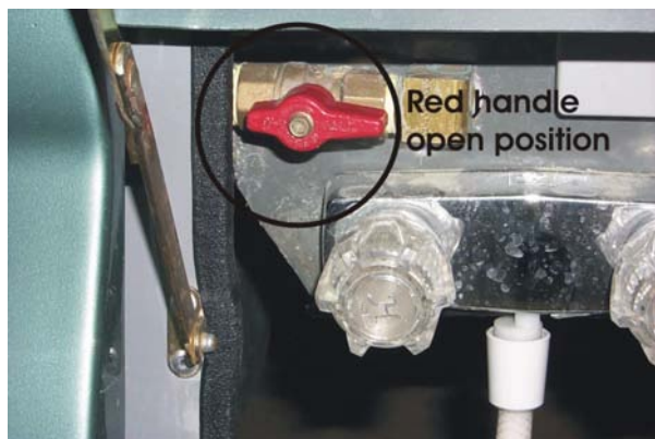
👉 Picture G-P3: Open position of the city water tank fill shut off valve.
