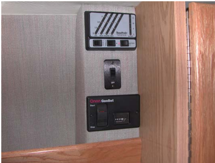
Picture E-P1: Monitor panel, porch light and optional generator on / off switch.
