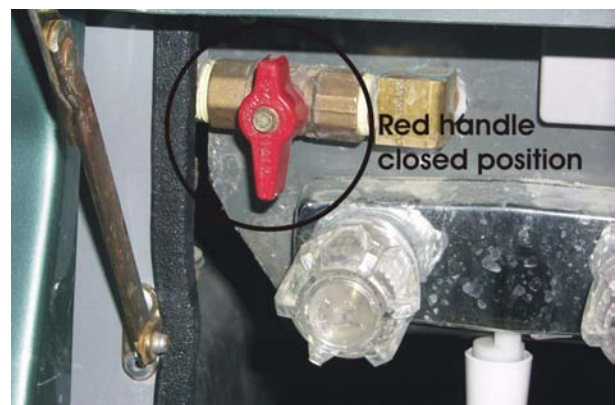
👉 Picture G-P4: Closed position of the city water tank fill shut off valve.
