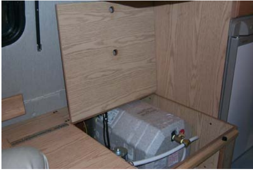
Picture G-P16: Water heater access door.
