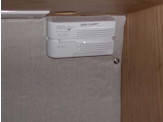
Picture F-P2: Carbon monoxide leak detector.
