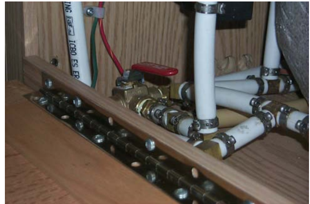
👉 Picture G-P15: Tank selector valve location. Valve is in the interior tank position.
