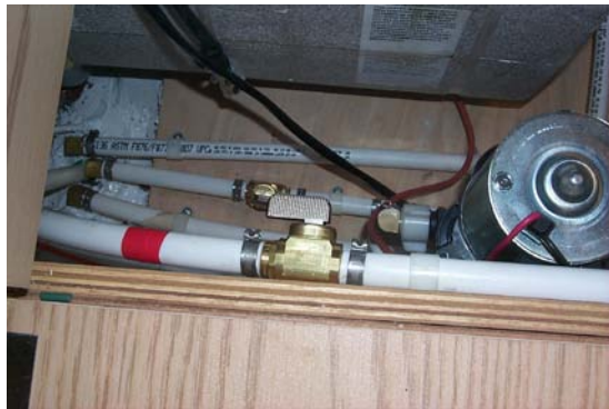
Picture G-P18: Hot water cutoff valve in open position.
