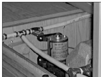
Picture G-P17: Water heater access door.
