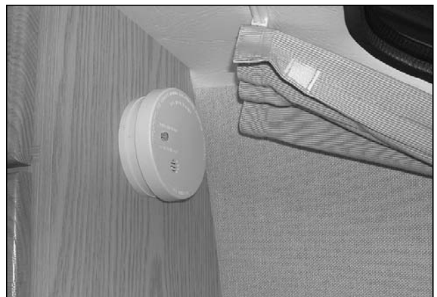
Picture F-P4: Smoke detector.
