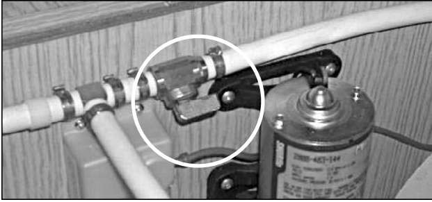
Picture G-P19: Hot water cutoff valve in the open position.
