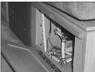
Picture G-P16: Location of the access door for the fresh water selection tank valve, (190 model).
