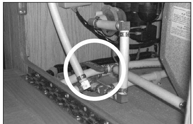
Picture G-P13: Selector valve supply from the interior fresh water tank, (winter position 190 models).
