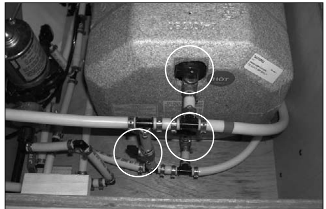
Picture G-P15: Winter mode, water heater by pass valve positions.
