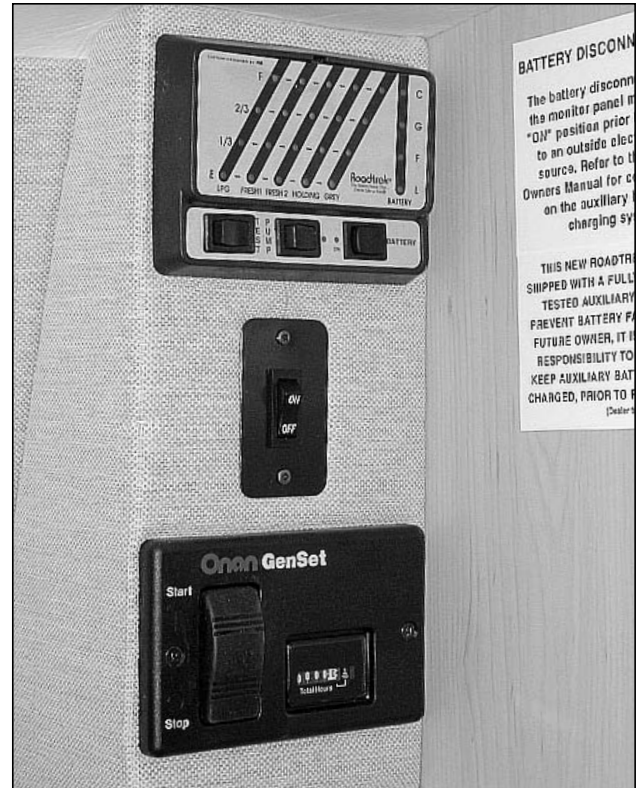
Picture E-P1: Monitor panel, porch light and optional generator control switch.
