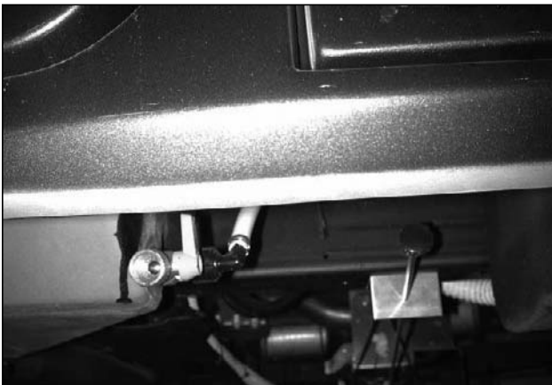
Picture B-P43: Exterior fresh water drain valve and macerator manual crank handle, 190 model shown.
