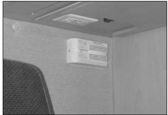
Picture F-P2: Carbon monoxide leak detector.
