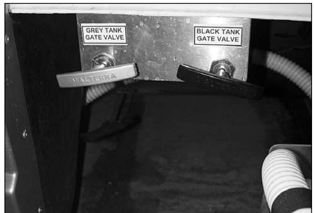
Picture G-P14: Access to sewer discharge assembly, black and grey gate valve handles.
