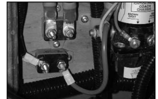
Picture B-P26A: Power Sofa 30A breaker
